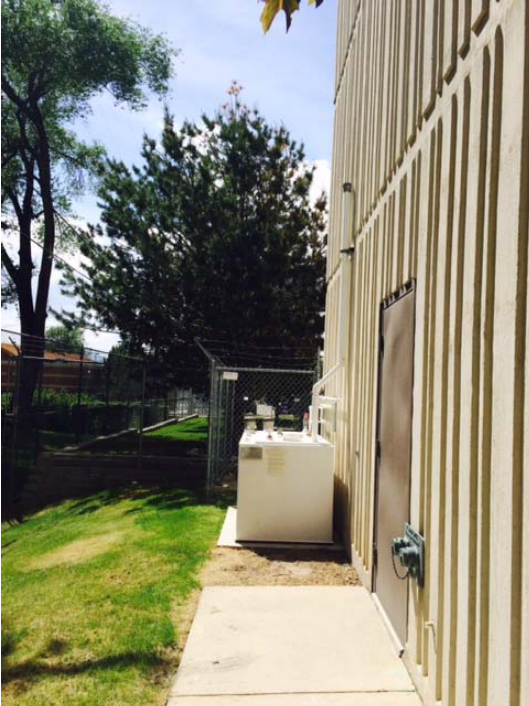
Looking towards the west, at the south façade of the Phillips Plaza Apartment Building. The generator would be placed to the left of the existing generator which is shown in this photograph.
